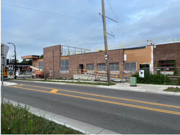
Pictured right: North addition from Penn Ave. The exterior envelope will be finishing in August. This building will house additional NorthPoint services.
