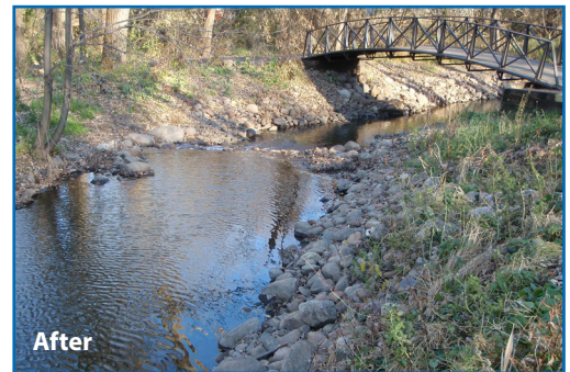
Hennepin County awarded the City of Golden Valley $135,000 in 2009 to stabilize eroded banks along a 5,100-foot reach of Bassett Creek. Funding came from the county's riparian restoration and streambank stabilization program, which received $500,000 from the Minnesota Clean Water Fund.
